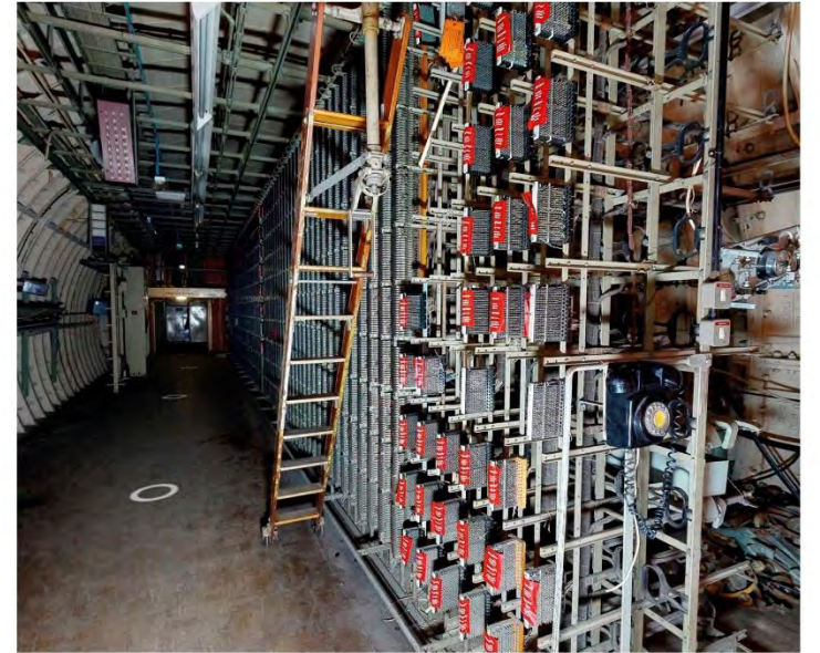
6 Telephone Main Distribution Frame
